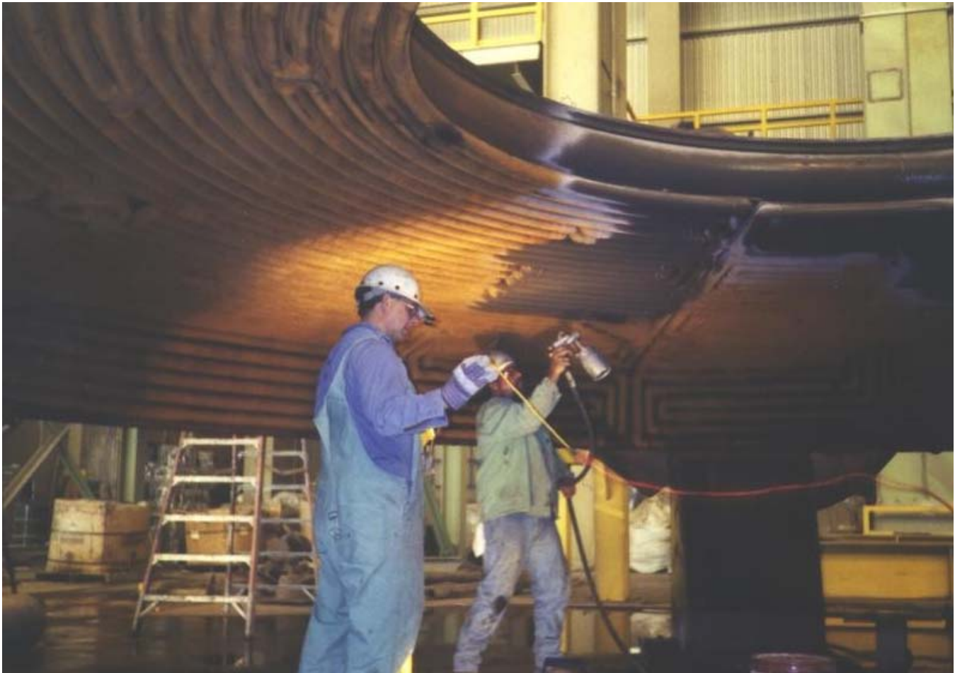
Figure 5 – Application of high temperature high emissivity coating to a water panel EAF roof
